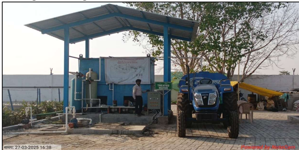
Carbon Filter and Clear Water Tank
