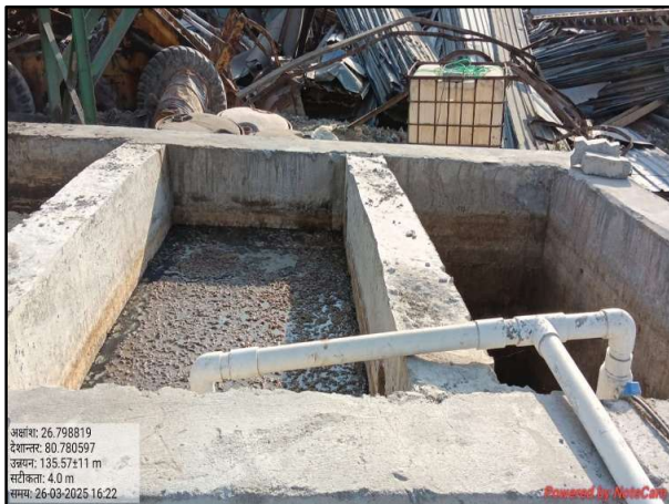
Settling and Sludge Tank
