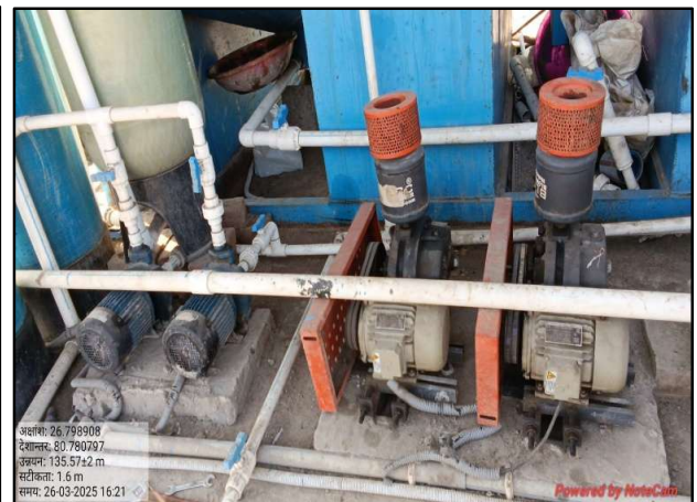
Pump and Blower
